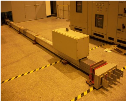
Clause 8.2.4.2 : Verification of effectiveness of the Protective Circuit (Icc) – Feeder Elements without Tap-off Unit
