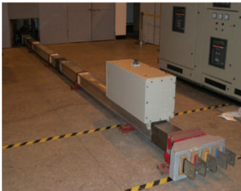
Clause 8.2.3.2.3a : Verification of Short Circuit Strength (Icc) - Feeder Elements without Tap-off Unit
