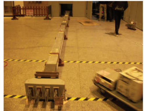
Clause 8.2.4.2 : Verification of effectiveness of the Protective Circuit (Icw) – Feeder Elements without Tap-off Unit
