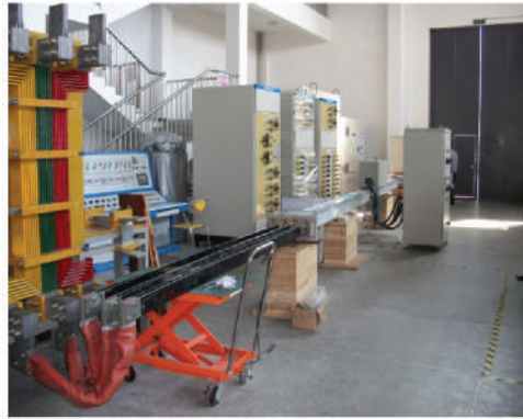
Clause 8.2.1.3b : Verification of Temperature rise Limits – Feeder Elements with Tap-off Unit
